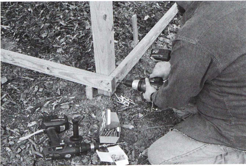
All fasteners exposed to the weather must be weather resistant, galvanized, zinc-coated brass or stainless steel.
