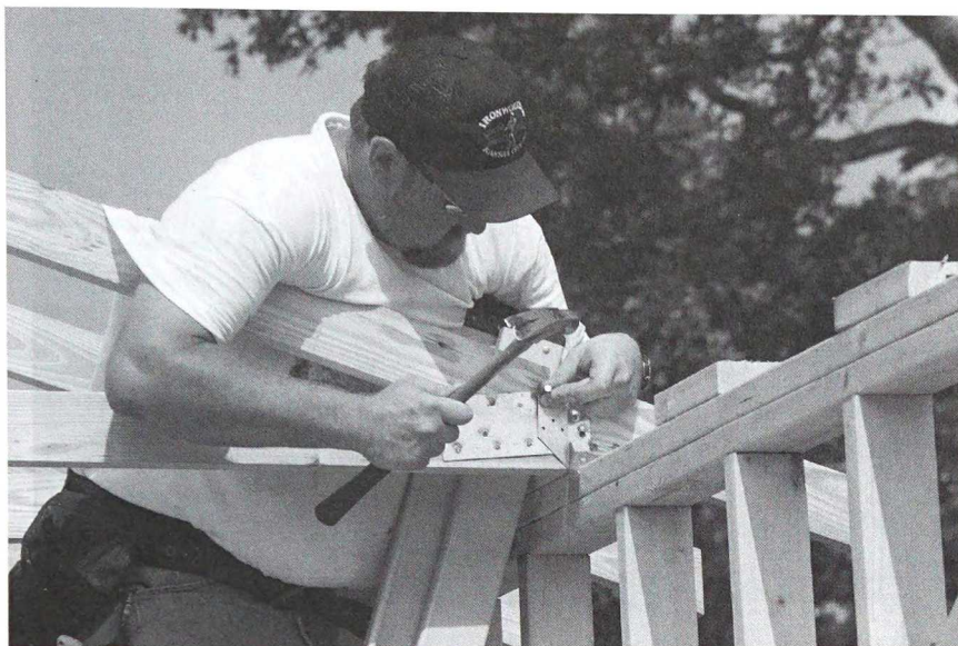
Truss hangers, or hurricane strips, and toenailing into the truss stop blocks is used to anchor the truss ends.
