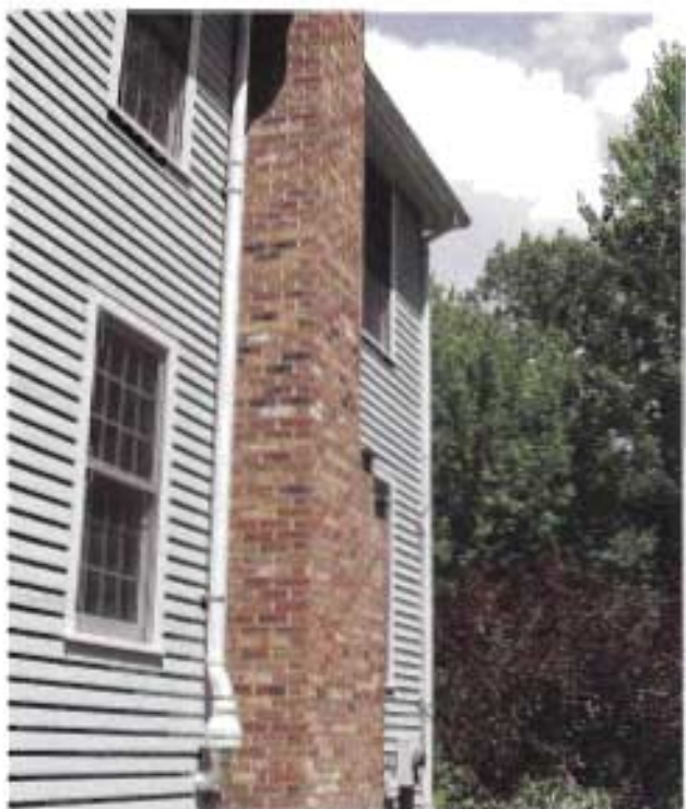
One form of radon mitigation involves installing a vent pipe to pull this harmful radioactive gas out of your home.
