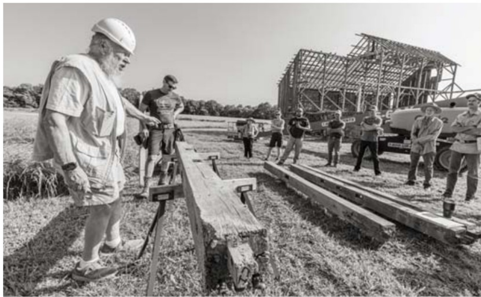
Restoration of the Colburn Barn began with a week-long course on timber frame construction.
