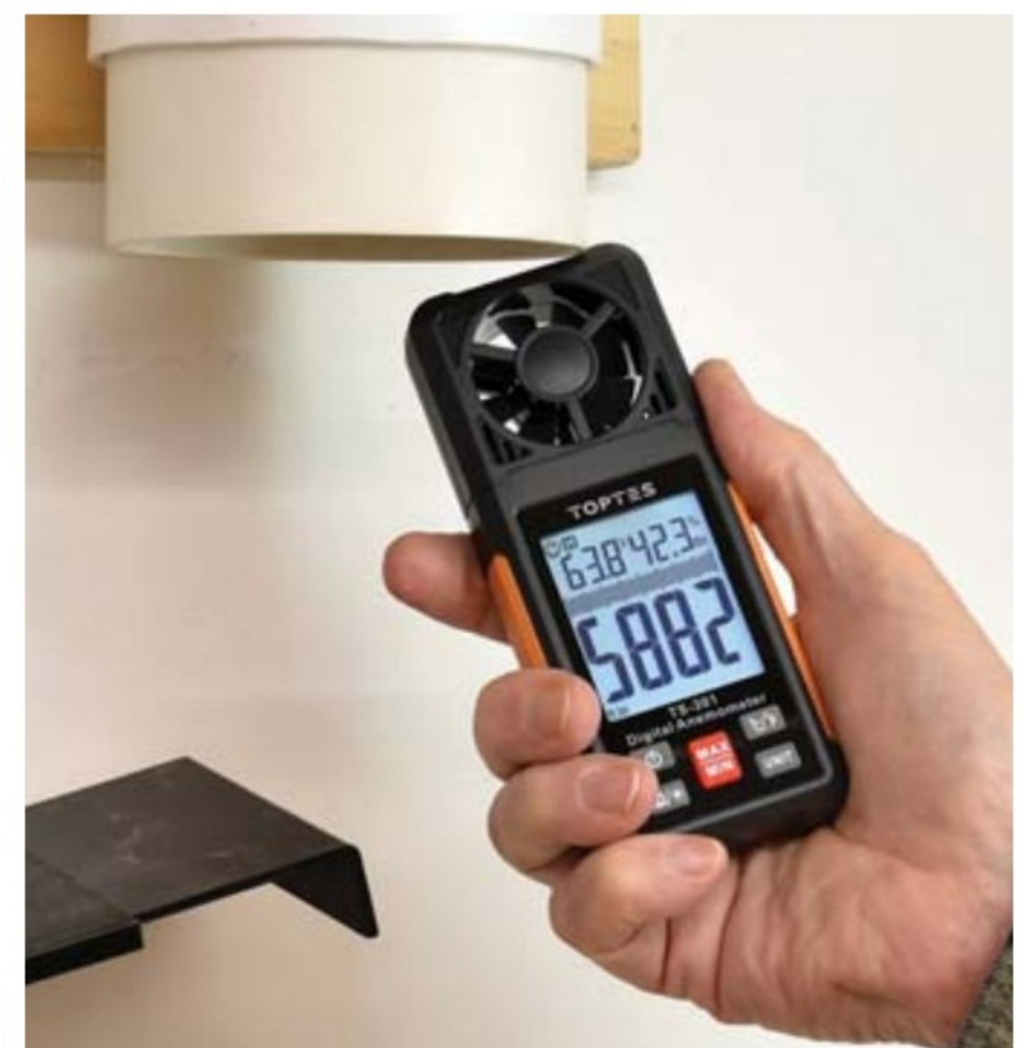
A handheld anemometer can show airflow rates at specific points in a duct run. Here the connection at a miter saw connection shows 5,882 ft/min, which converts to about 513 cfm.
