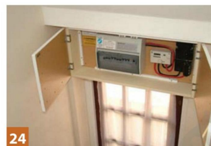
24 The meter-covering cupboard with the doors added
