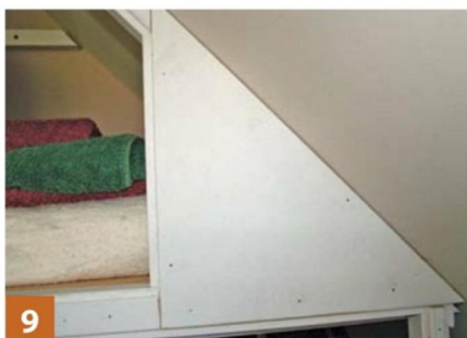
9 MDF panels cover the areas which do not have doors
