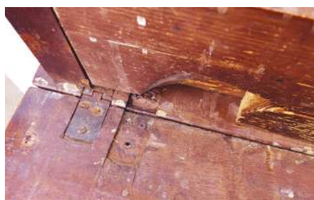
The original hinge position where the screws must have pulled out
