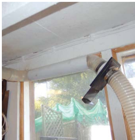
It is quite easy to install a small extraction system of pipes and branches that reach all machines
