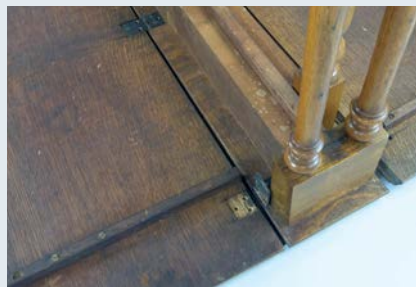
Loose hinges where the screws had pulled out of the timber
