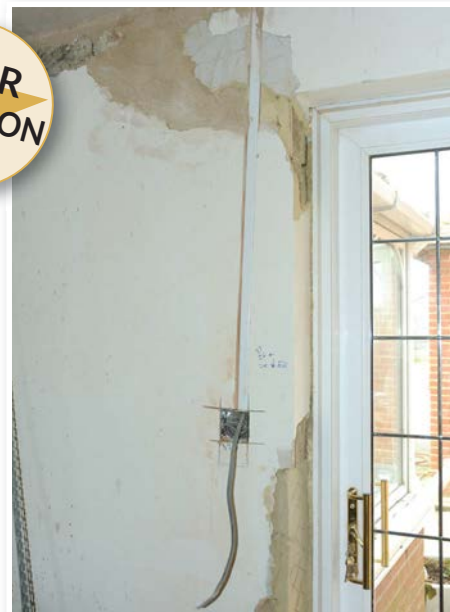
Repair to mortar and plasterwork where cracks have occurred next to a uPVC window. Timber joinery causes less disturbance to the surrounding structure
