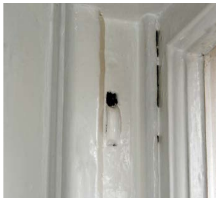
This sash window has seen better days but it can be put right again
