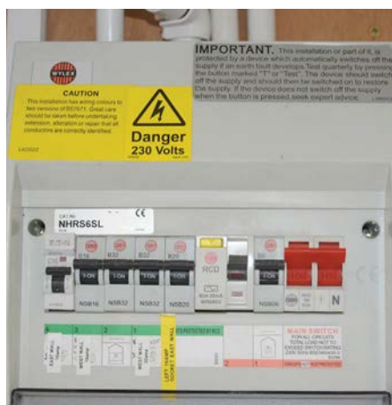
Modern consumer units can shut off if earth leakage due to moisture is detected
