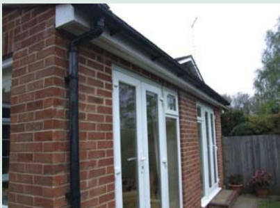
An extension uses plastic covering fascia and soffit
