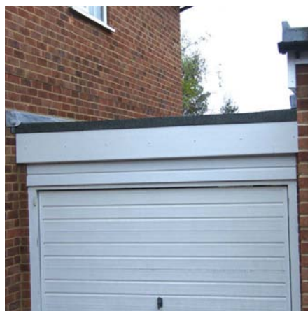
This shows an example of plastic covering used over the timber at the front of a garage
