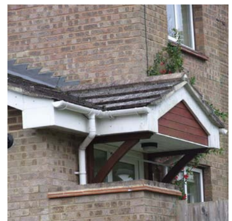
Porches are among the structures that can make use of plastic covering over the barge boards, fascia and soffit
