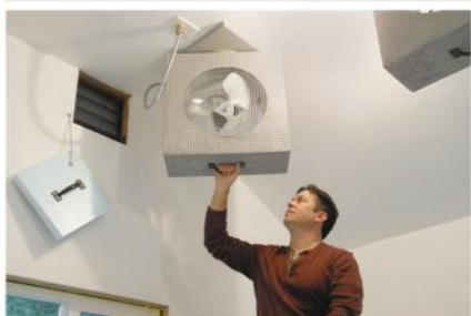
The author attached his fans to a lazy Susan to make reversing the airflow easier. Note the vent in the wall and the foam cover for the vent.
