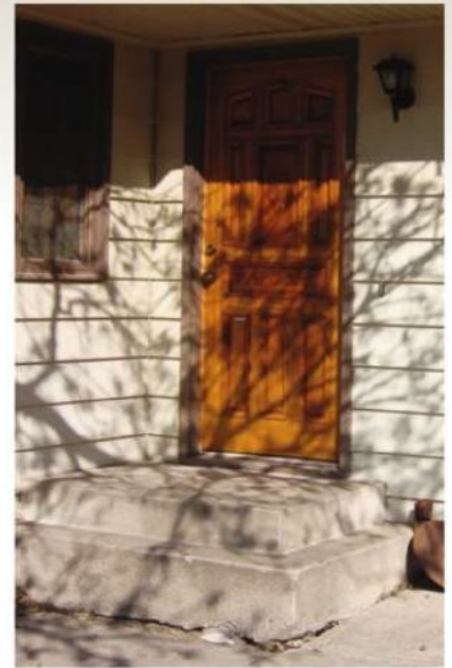
Aging concrete steps did nothing to enhance the beauty of a new screen door project, but removing the old steps wasn't an attractive option either.
