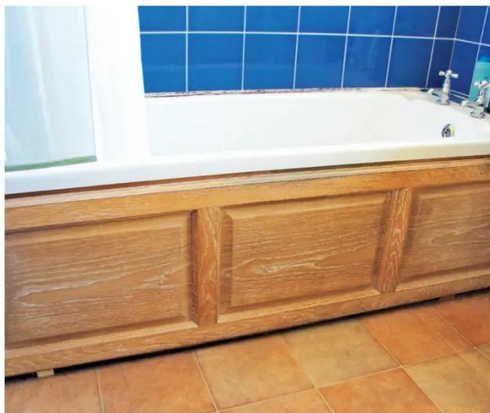
1 The existing bath panel looked tired and supporting framework suffered from water damage
