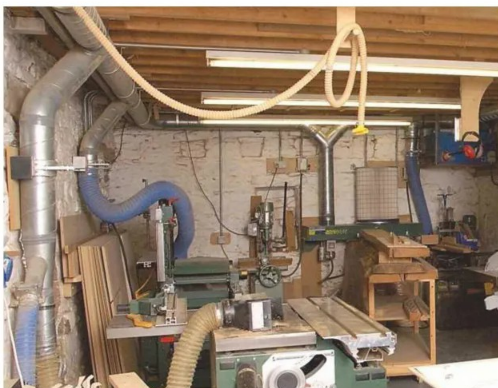
9 A collection system around the workshop, using metal ducting, minimises airflow resistance and avoids electrostatic problems
