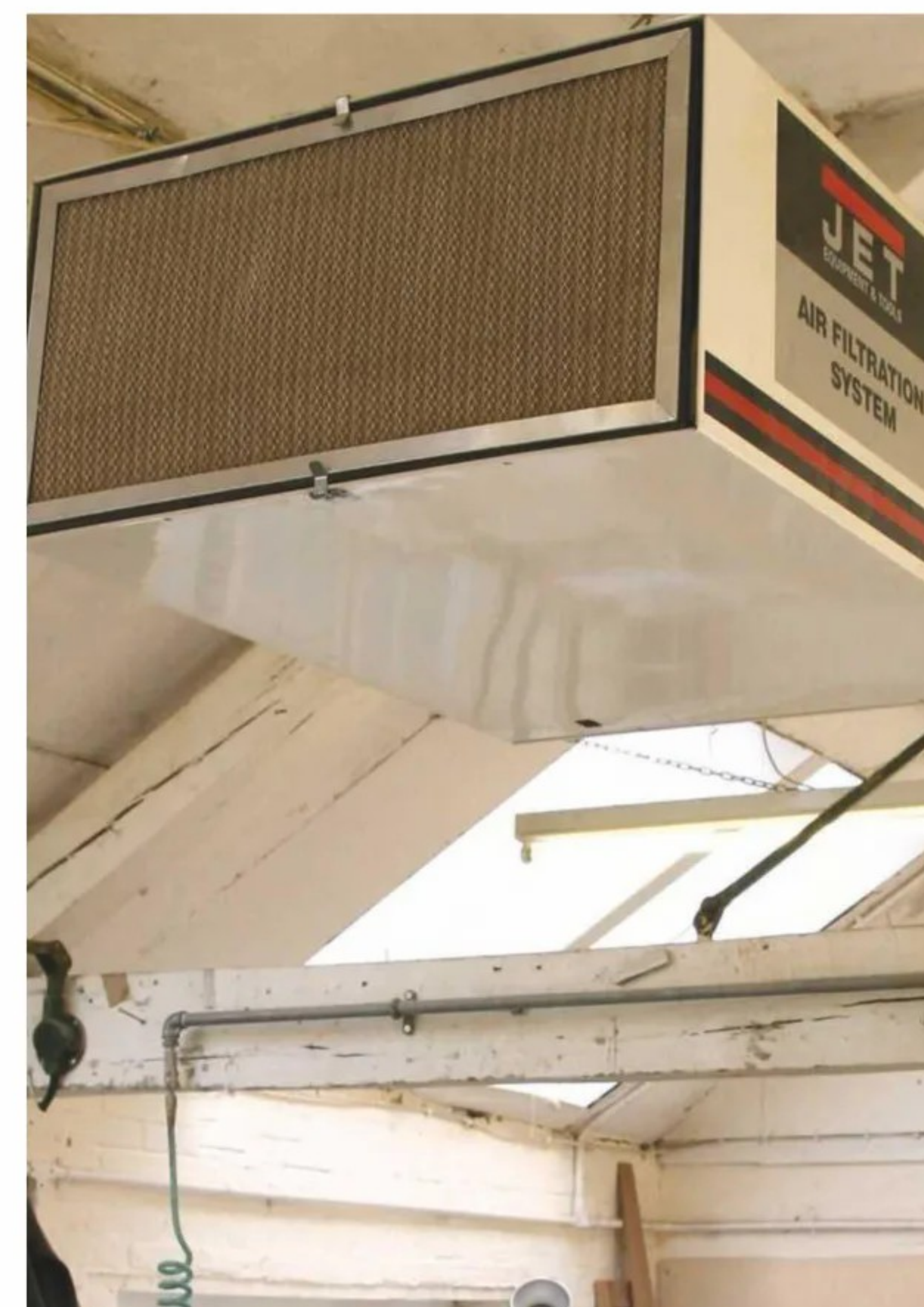
15 Air filtration systems clean floating particles of fine dust – the most damaging kind – by catching them in electrostatic filters
