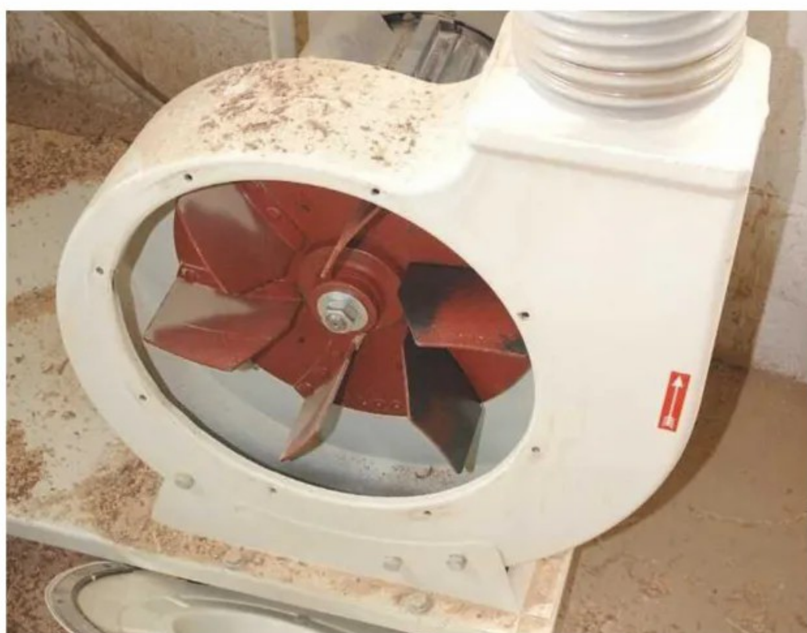
10 The centrifugal fan on a high volume extractor passes wood chips, along with air, into dust collection sacks
