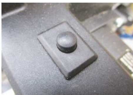
No label for the lighting switch
