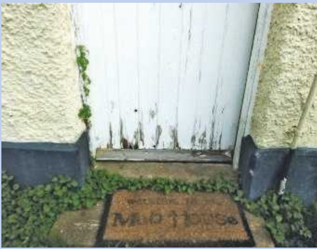
2 Bottom of door showing extensive rot
