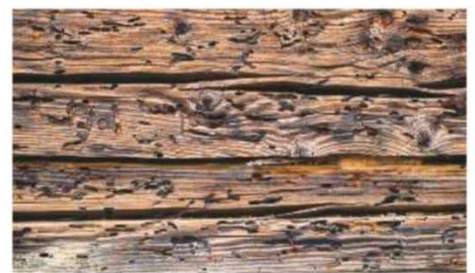
Termite damage in wood
