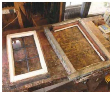
2 Stripping paint = fire!
