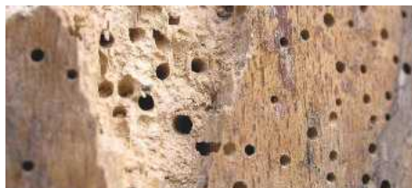
Wood-boring beetle holes
