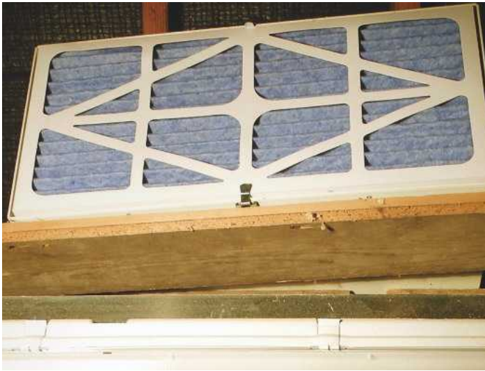
9 An ambient air cleaner sucks in dirty air and returns it, cleaned, to the machine 'shop
