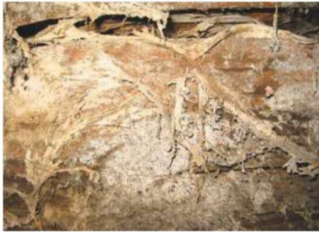
Wooden beam with significant fungal growth
