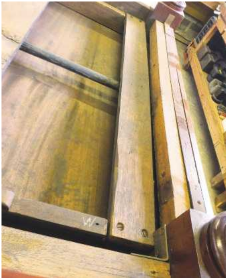
2 There were breaks, battens and bits of metal all over the frame
