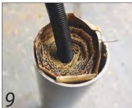
9 Steam goes in at this end
