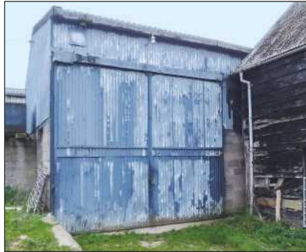
What's behind these doors?
