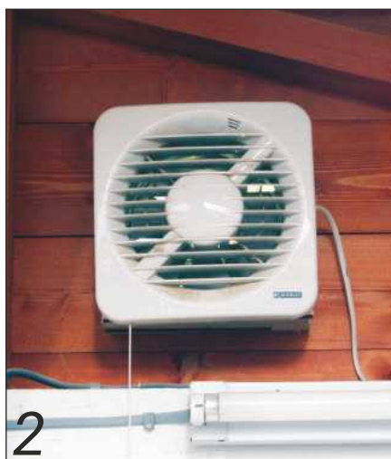
An extractor fan is inexpensive and removes contaminated air from the workshop very quickly. In summer it also encourages a flow of cool air through the workshop, but in winter it removes warm air as well as dust
