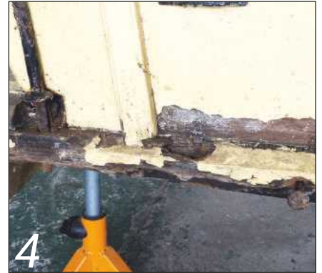
4 On one corner, the wood had rotted away around the metalwork
