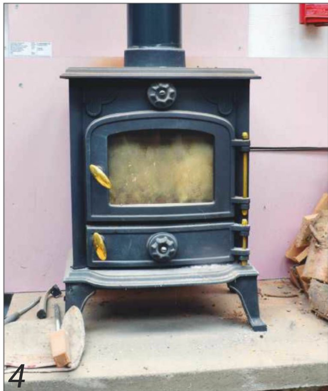
My woodburning stove is mounted on a stone slab with a double layer of fireproof board behind it
