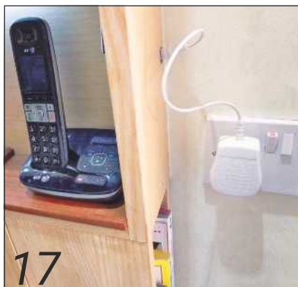
17 The supply socket for the lighting is lower down on the wall beside the cabinet
