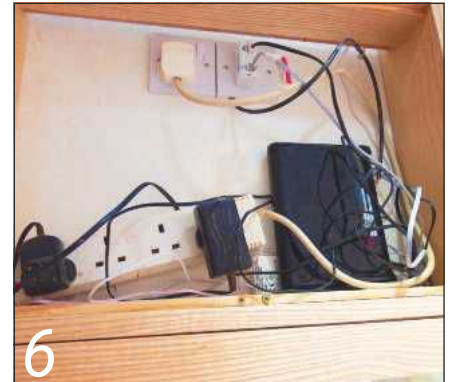
6 The top is vented via a gap at the back to allow any heat from the transformer plugs to escape
