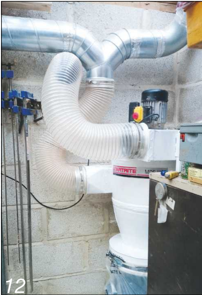
12 Using a ducting system, the airflow is moved directly out of the workshop
