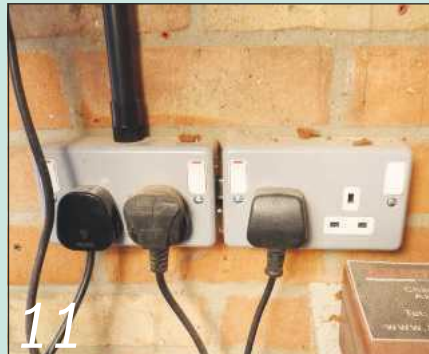
11 Metal-clad socket outlets are much more suitable than plastic ones in a workshop. I made sure I had plenty of them
