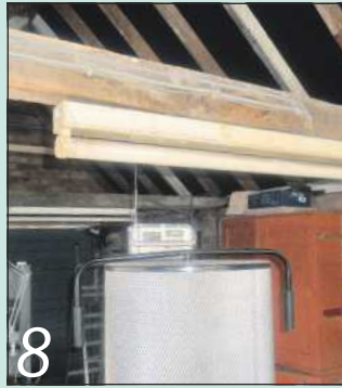
8 The existing lighting was provided by a couple of low and unprotected fluorescent tubes
