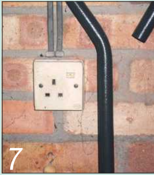
7 The machine shop electrics consisted of a few plastic power points in all the wrong places
