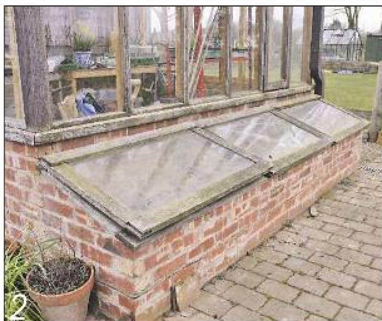
2 The oak has now weathered and turned grey, and the joints have failed
