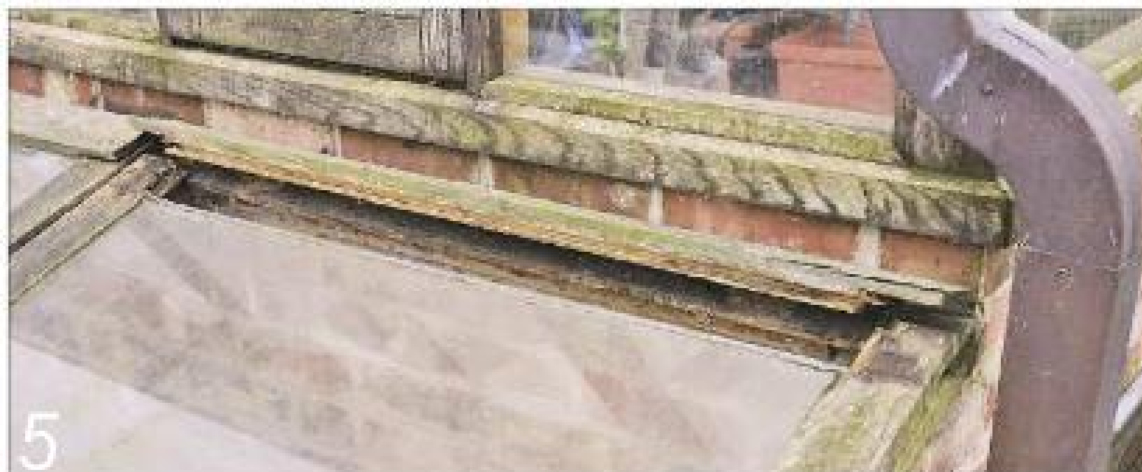
5 The joints on the hinge rail were the most stressed and have literally fallen apart
