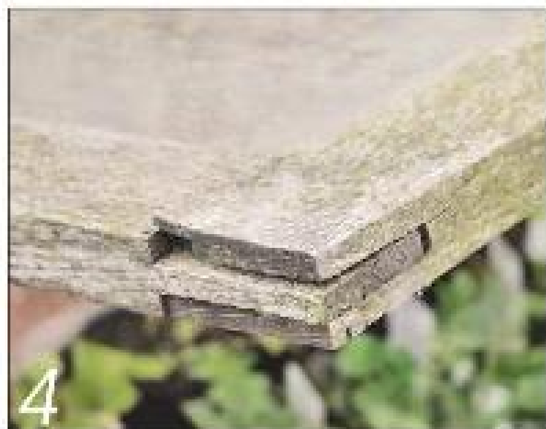
4 The corner bridle joints began to open up along the glue line many years ago
