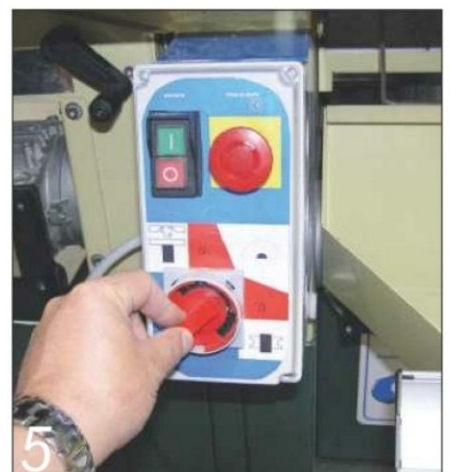
Central switching is usually standard for isolating each motor function
