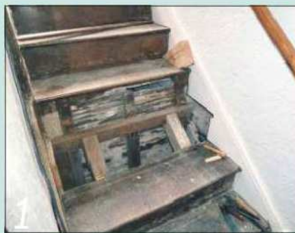
1 We couldn't work out what had been holding these treads up, as it looked as if there had never been any supports
