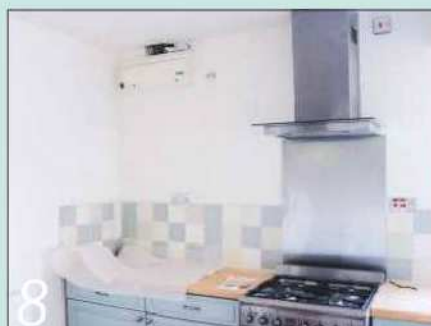
8 As you can see, the wall hanging brackets for the cabinets are directly in line with the opening flap on the consumer unit
