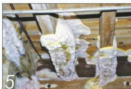
5 The most dangerous fungi of all, such as the dreaded dry rot, attack wood while it's in service
