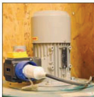
The substantial Siemens motor and NVR switch
