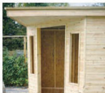
24 The door and window framing is fitted proud of the cladding
