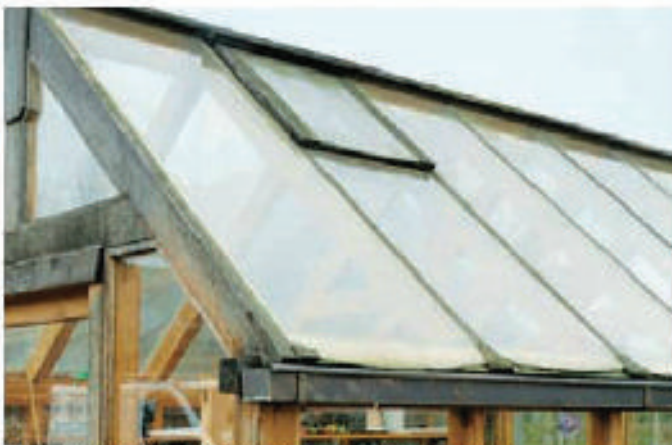
2 The joints on my greenhouse tanlight failed within three years – a very poor performance over such a short timespan
