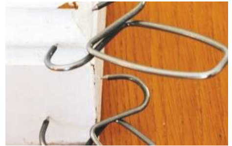
Here, clamps span the joint and apply pressure to this skirting mitre
