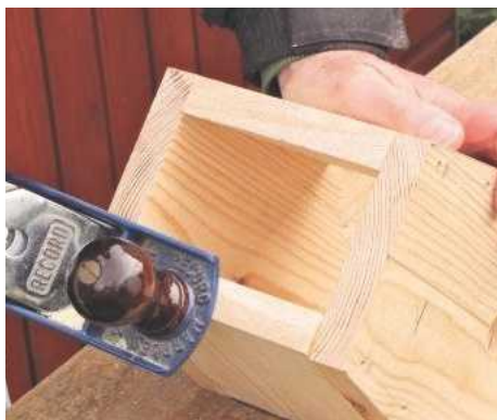
7 Trim lower edges flush with a plane, working in from the ends towards the middle to avoid breakout
