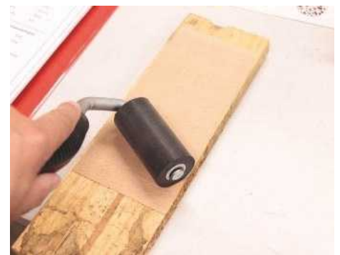
... and once on the substrate, apply pressure with a 'J' roller to ensure a good bond
