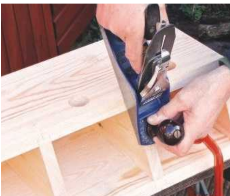
10 Check top edges are flush, trimming with a finely-set plane if necessary; tidy up internal arrises
