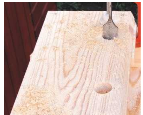
6 Mark centres and bore 32mm holes with a flatbit, remembering to clamp the offcut underneath
