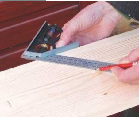
1 Mark out the front and back sections using a combination square; the roof is pitched at 45°
