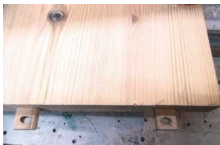
6 Dowel holes enlarged for movement
