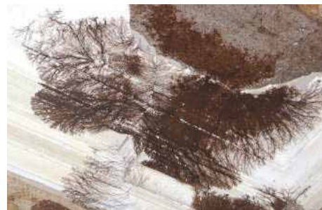
Wet rot attack
