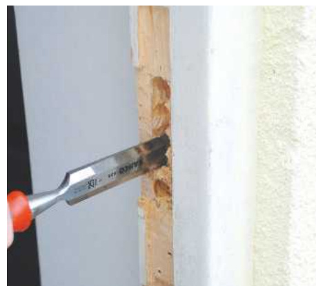
20 Remove most of the waste with a drill and flatbit, tidying up the mortise with a chisel. You can then refit the striker box
