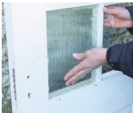
22 Add putty around the inside of each rebate and press the glass into place
