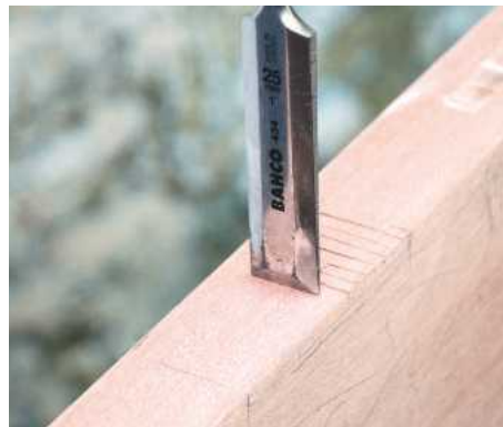
10 Either use a router to cut the hinge recesses or chop them out with a wide chisel. Check recesses for depth
