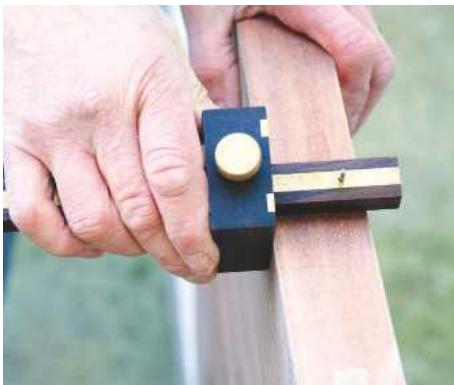
9 Screw new hinges to the jamb and re-position the door. Mark their positions on the door and set the gauge to flap width
