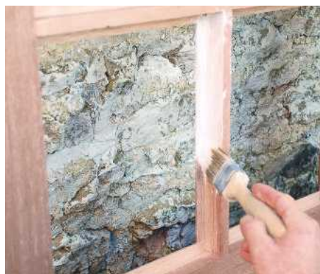
7 Remove the beading strips. Paint all rebates and rear edges of the beads with an oil-based primer
