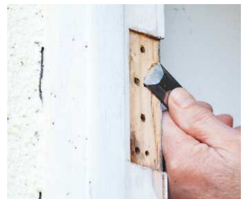
8 If re-using existing hinge recesses, pare cleanly with a chisel. Plug holes that don't match new hinges
