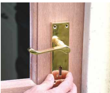
12 Decide on lock height and check both handles. Try to avoid cutting into the middle rail joint
