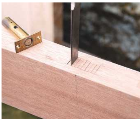
21 Mark the position of the concealed bolt, chisel out, then bore a clearance hole. Next, drill a hole for the key on the inside face of the door
