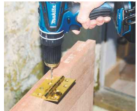
11 Position hinges and use a bradawl to mark the centres on each flap. Drill and screw both hinges to the door
