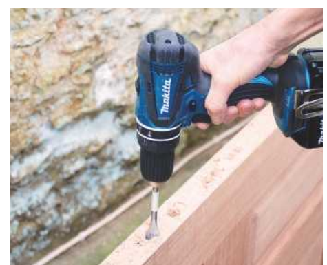
14 Bore overlapping holes to suit lock thickness along the edge of the door. Use a flatbit or auger bit with masking tape
