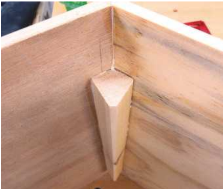
21 I cut the top edges of both roof panels at 30° and glued and screwed these to the ridge piece after carefully marking its position
