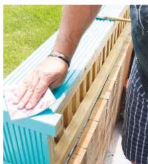
The base coat is de-nibbed with a fine abrasive and dusted off
