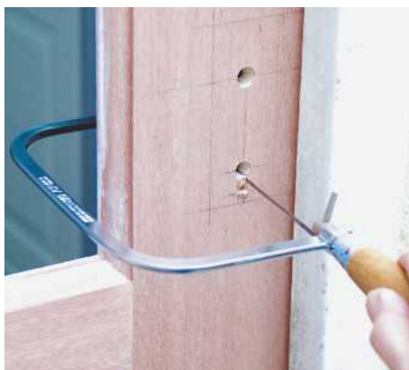
18 Drill holes for the spindle and keyhole, working from both sides of the door. Enlarge the keyhole with a coping saw
