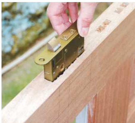
16 Check the lock is a snug fit in the mortise. Carefully draw around the faceplate to give an accurate line for the recess corner
