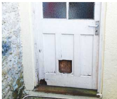
1 The existing door was beyond repair, with an unused cat flap cut-out and serious rot at the bottom
