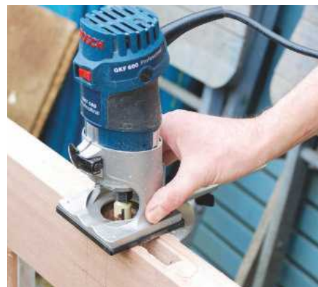
17 Carefully cut the lock recess, using either a small router or chisel. Trim the ends square if necessary
