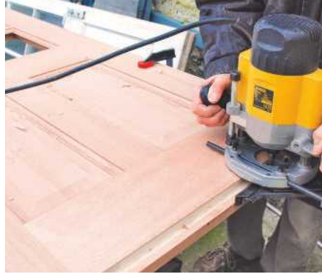
4 Rout a suitable rebate along the door's bottom edge to clear the water bar in the frame's threshold
