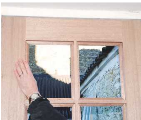
6 Next, position the door in the frame and check it's not too tight. Aim for a 2.5mm gap along each edge
