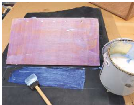
23 Having marked the rubber roof covering with white marker pen, I then applied the glue
