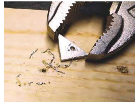
18 Once all the triangular splines have been cut, drill a small hole in each at the point where it'll be inserted into the box
