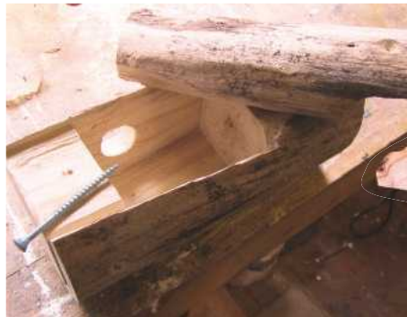
10 The screws going into the top – on the left of the photo – were set well away from the end so that they wouldn't foul a sloping cut for the roof
