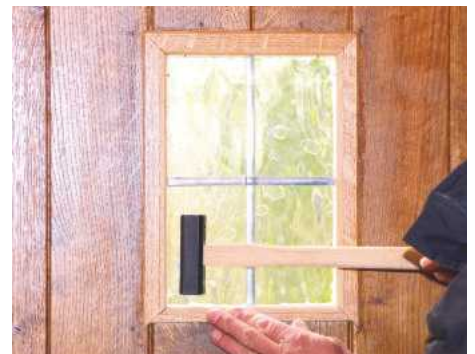
8 Fit oak beads to the glass around the inner frame. These are mitted and fixed with brass pins and sealant ✂
