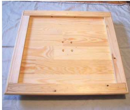
7 Holes drilled ready to screw the base to the lower end of the pillar
