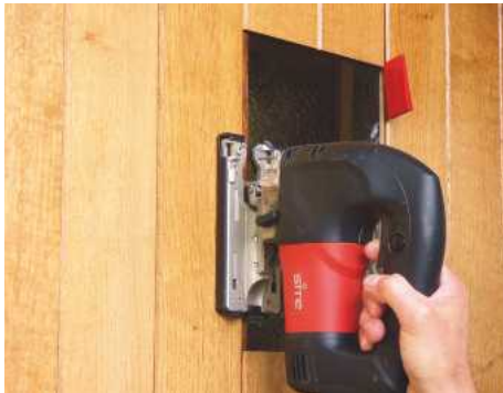
1 Carefully cut away sections of loose tongue on the matchboard using a jigsaw fitted with a fine blade
