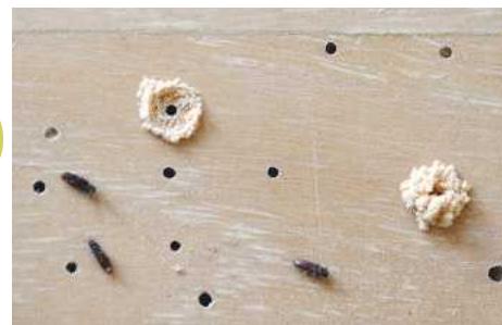
Powderpost beetles and damage shown to a wooden floor
