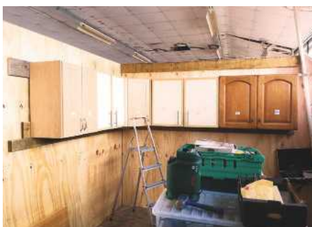
8 Typical cupboard installation
