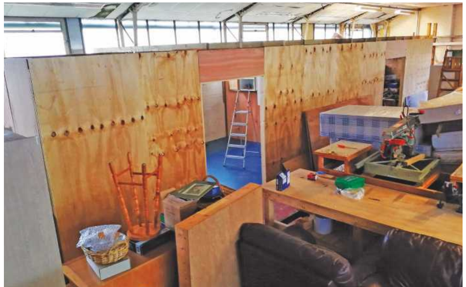
7 The most recent photo of the whole project, which was taken up a ladder to give an indication of room size
