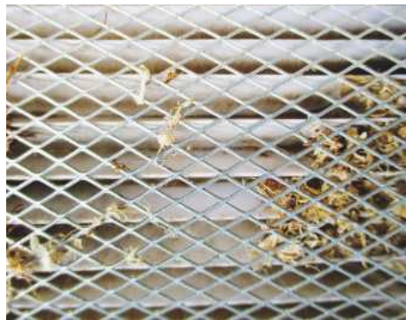
... but the HEPA filter will soon be blocked
