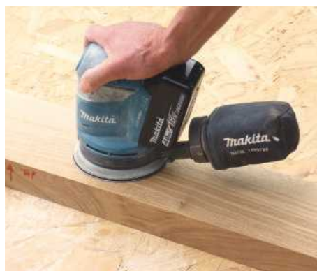
11 Sand all exposed surfaces with 180 grit abrasive. Lightly dampen the oak to raise the grain, then lightly sand again by hand
