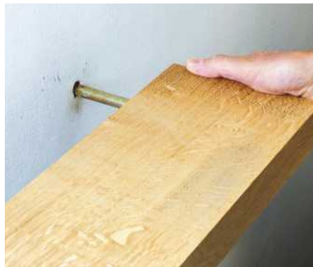
8 Slide the shelf onto the brackets, tapping gently from the front with a hammer. Make sure you use scrap wood to prevent denting the surface
