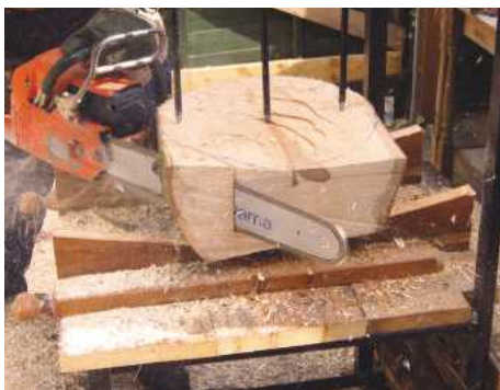
5 I secure the blank with an additional two spikes; this ensures there's no movement when I come to cut the cheeks off the blank to create an octagon
