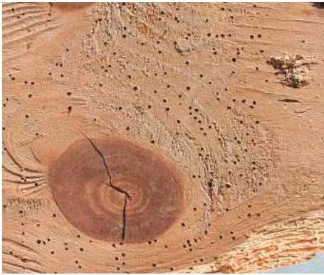
Signs of wood-boring insect infestation include 'frass'
