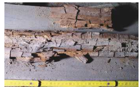
Wood decay caused by Serpula lacrymans (called true dry rot, which is a type of brown-rot)
