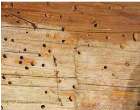
Damage left by wood-boring beetles
