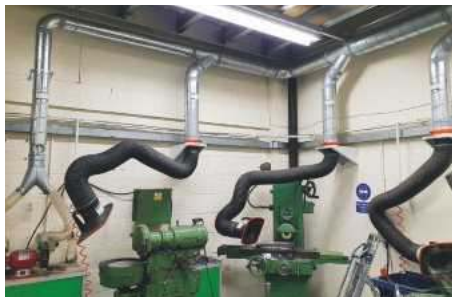
Dust extraction system on a more industrial scale
