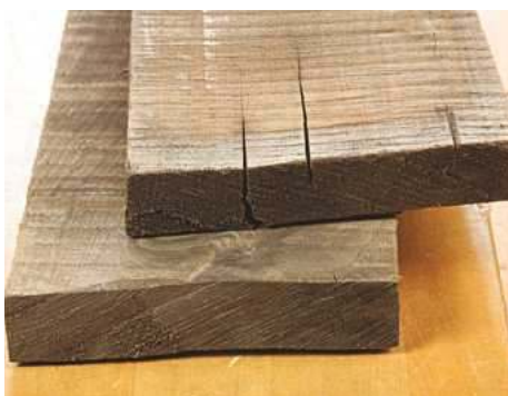
End checks in wood
