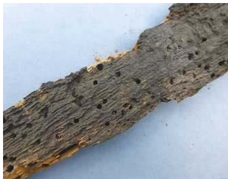
... and the damage it causes
