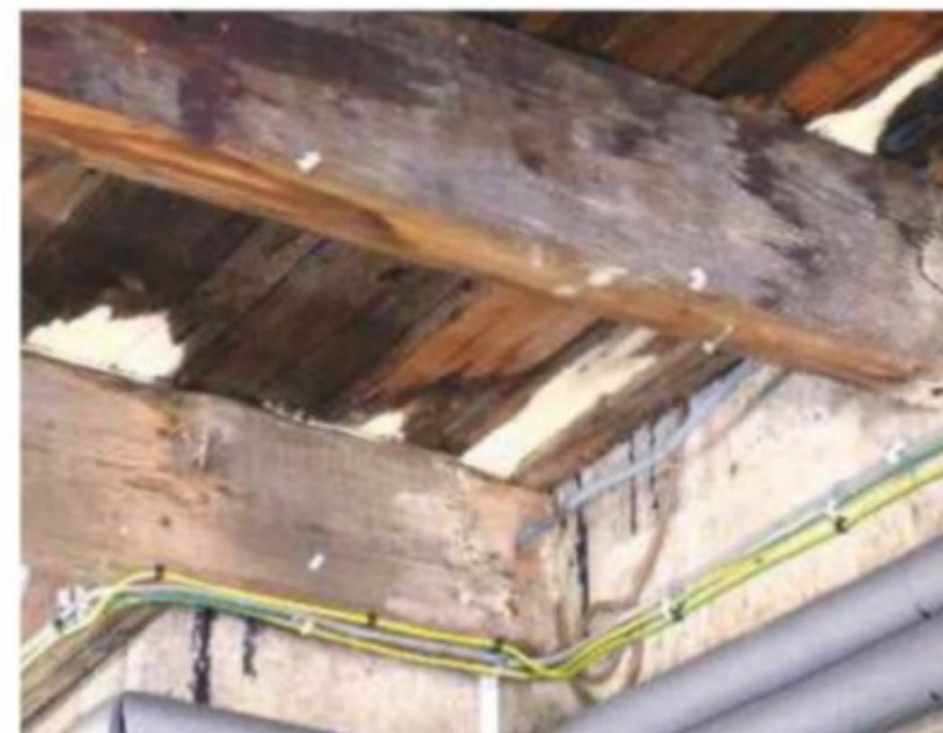
3 Water was coming in through the roof in several places, making it hazardous above electrical cables, light fittings and two consumer units
