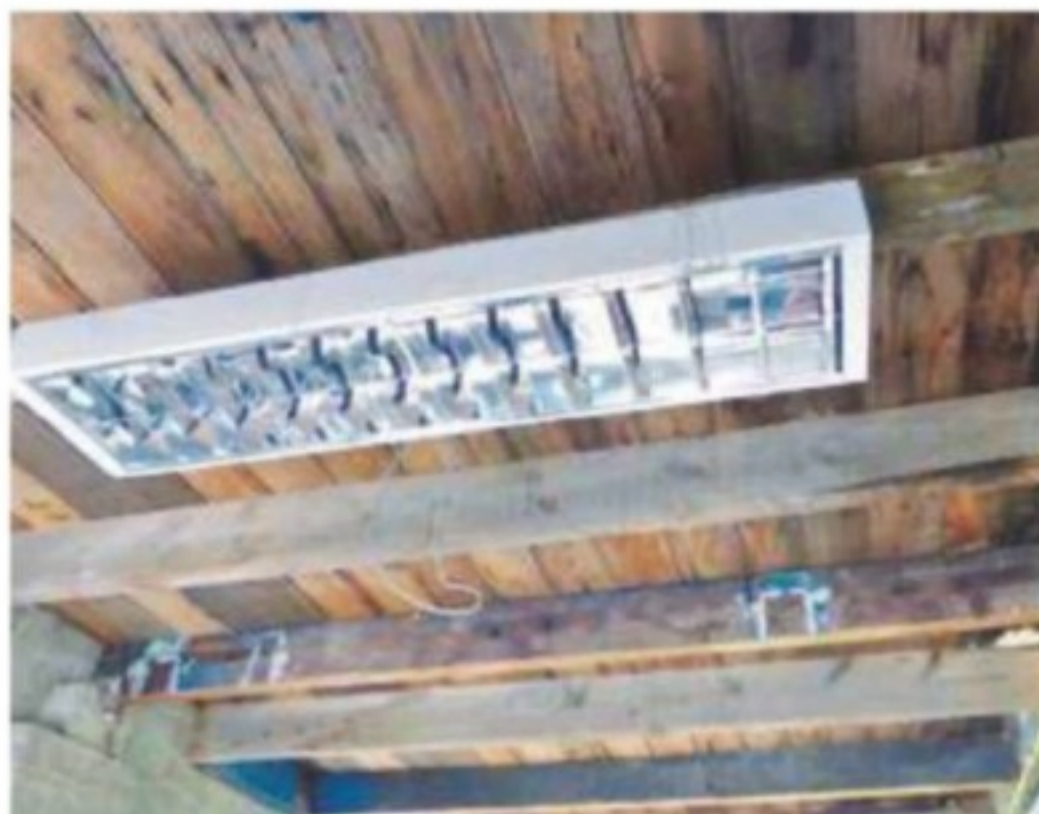
2 Although some of the old joists were sound, several had woodworm. Using second-hand timbers had certainly been false economy here
