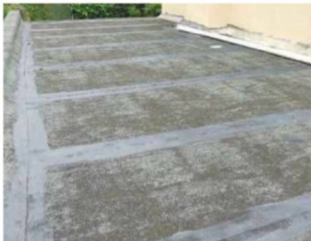
1 The bituminous felt on the existing garage roof was in a bad way, having cracked in several places. It needed replacing urgently before winter
