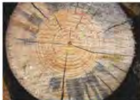
Blue staining on wood
