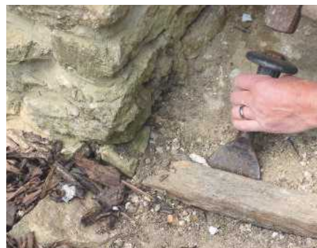
3 All rotten timber should first be removed. Here, the frame's threshold was sitting on bare soil, with no damp course at all
