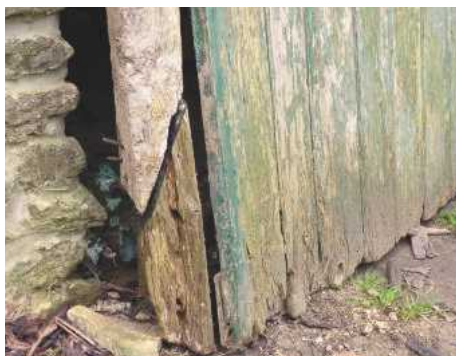
2 Although the oak frame had been repaired several decades ago, it had rotted badly. Both door and frame needed replacing
